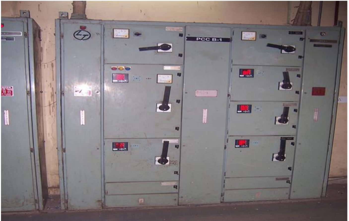
Fig 3: Photograph of Old distribution panel
