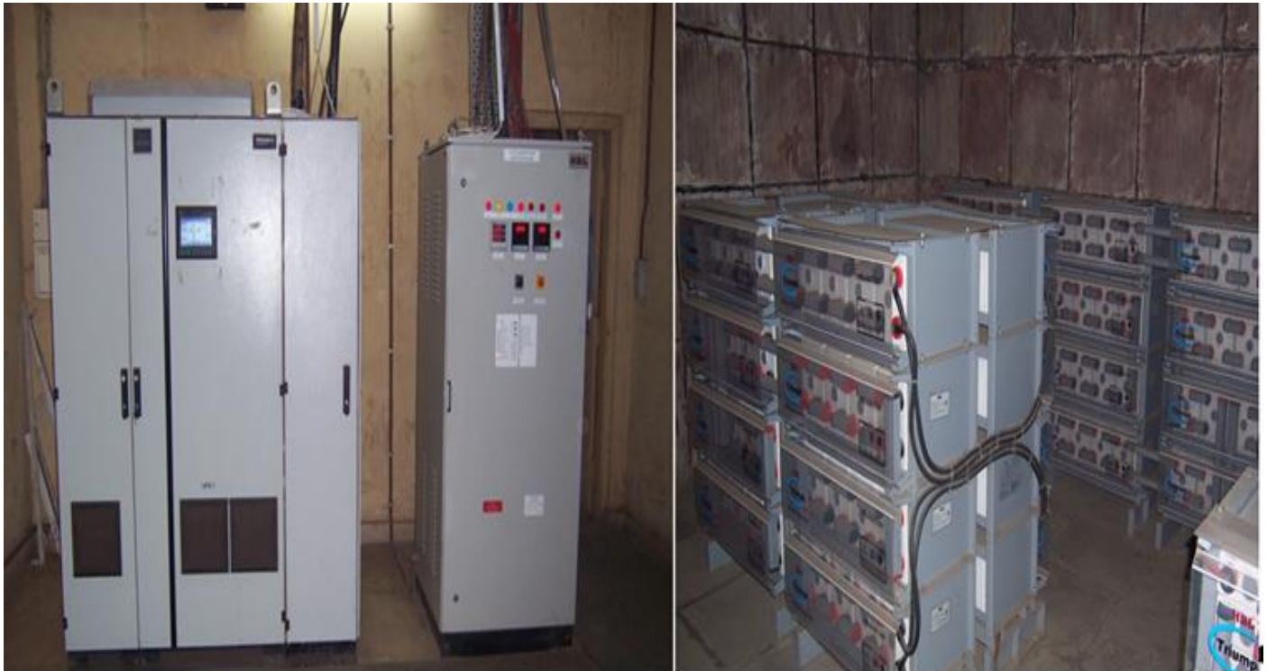
Fig 5: Photographs of the UPS and Battery charger system along with VRLA battery banks
