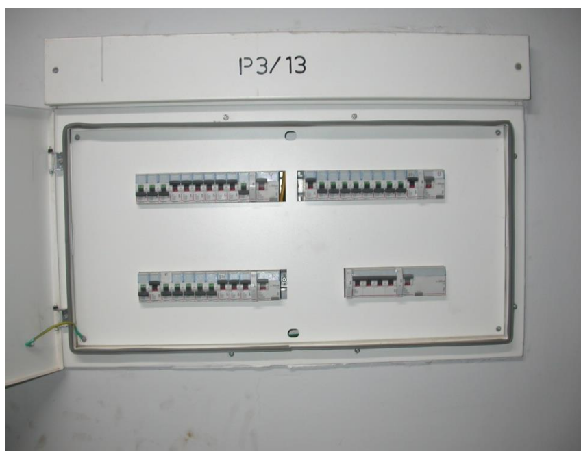
Fig 4: Distribution Board with MCB, RCCB and auxiliary contacts
