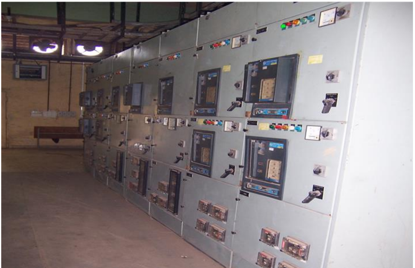
Fig 2: Photographs substation switchgears with circuit breakers
