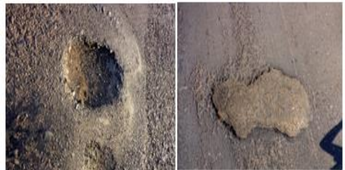
Fig 1:- Images of pothole surface
