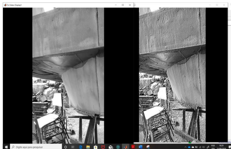
Fig 4:- Details of weld and deformation of vessel side
