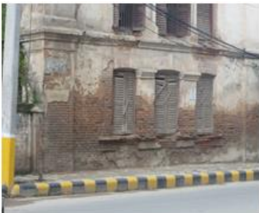
Fig 3:- Weathering of west wing outer wall
