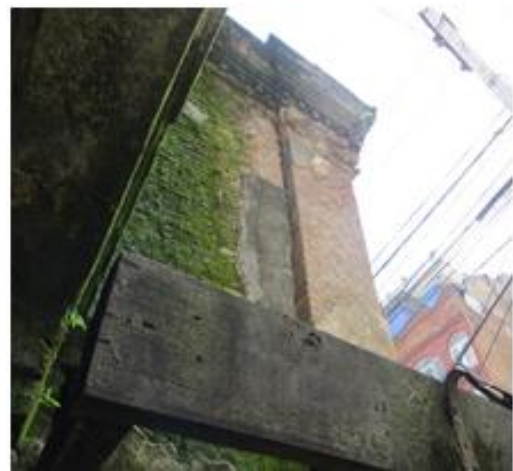
Fig 5:- Growth of plant in external wall of west wing
