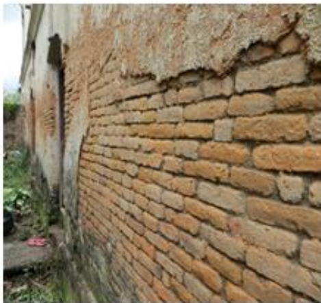
Fig 8:- Erosion of brick/mortar in external wall of North wing
