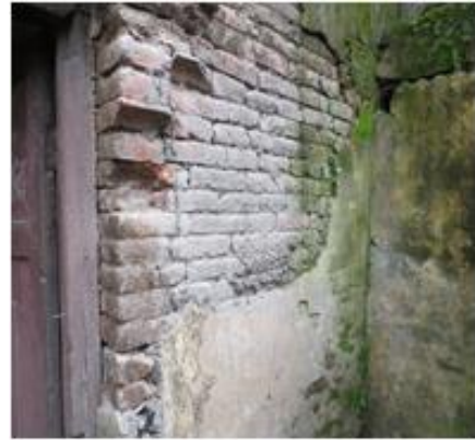
Fig 4:- Damages due to weathering of west wing outer wall
