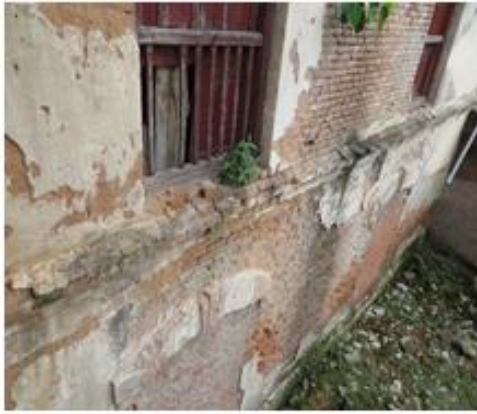
Fig 7:- Deterioration of brick of west wing outer wall
