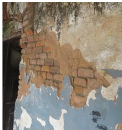
Fig 6:- Erosion of brick/mortar in external wall of west wing
