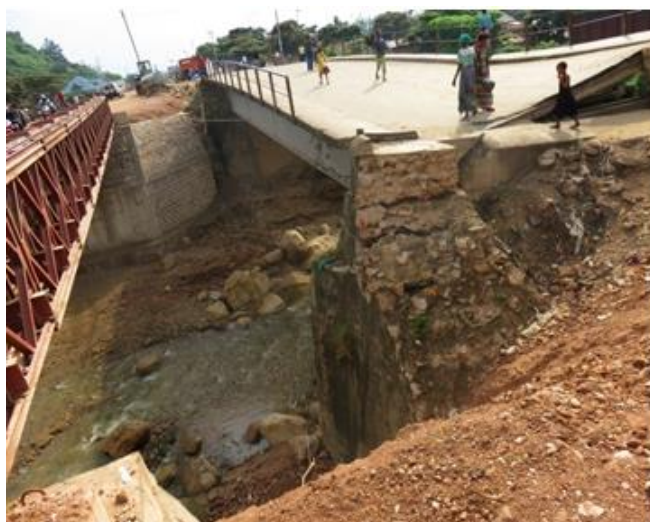
Fig 5:- Bridge collapsed on the RN5 on the right bank: (786m; 03 ° 21 '17,1lat. South and 029 ° 09' 15,8 East). This bridge was definitively damaged during a flood on the night of April 03 to 04, 2015. The RN5 serves the port of Kalundu on Lake Tanganyika: the country's second economic port after that of Matadi. Upstream of the destroyed bridge, a new erect
