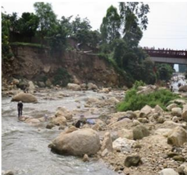
Fig 3:- Erosion on the left bank, upstream of the bridge: (03 ° 2115.3 lat. SOUTH and 29 ° 0914.4 Long. East). Shore at major risks. These houses, threatened with destruction, were established on this shore not 10 years ago. The population settled on this site for a permanent and regular supply of river water.
