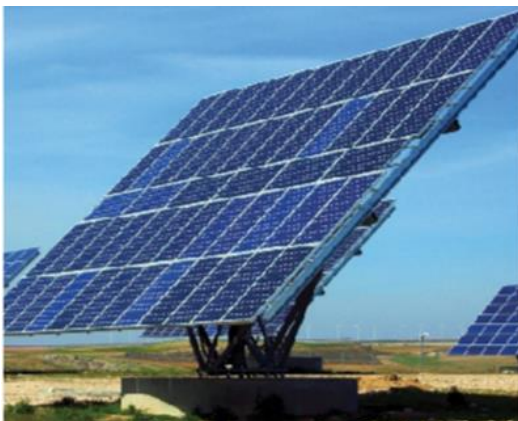
Fig 2:- Tracker-based solar array
