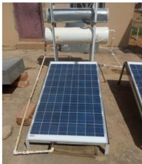
PV with cooling system
