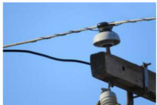
Fig. 2:- Electrical Conductor Placed on a Pin Insulator in the distribution lines.
