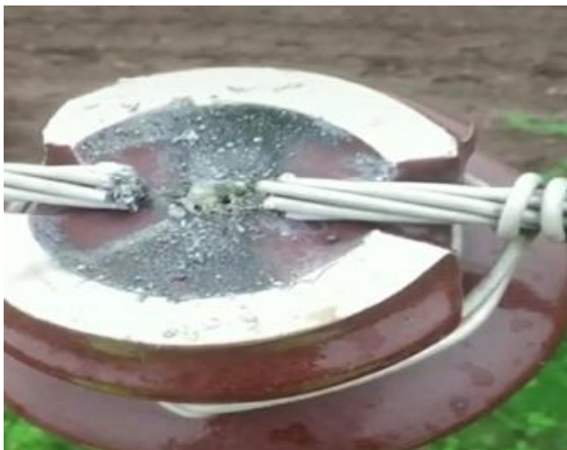
Fig.4:- shows the condition when the damage taking place to the Pin Insulator after fault.
