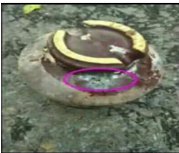
Fig. 5:- shows the condition after the fault when the Pin Insulator is fully damaged due to its exposure to the atmospheric conditions.
