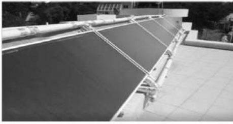
Figure 11.6 Solar panels over the roof tiles.
