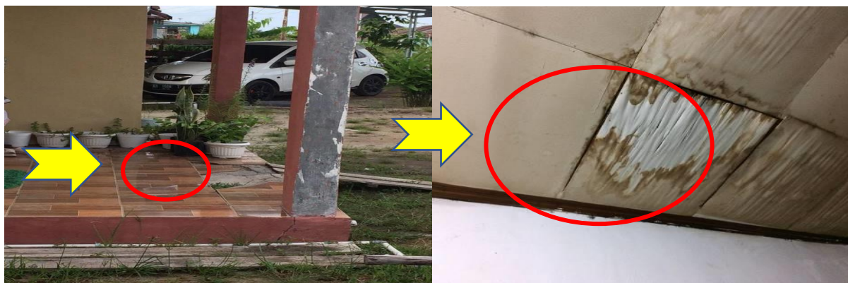
Fig.3. Damage on the floor tiles and ceiling in Borneo Sejahtera Resident
