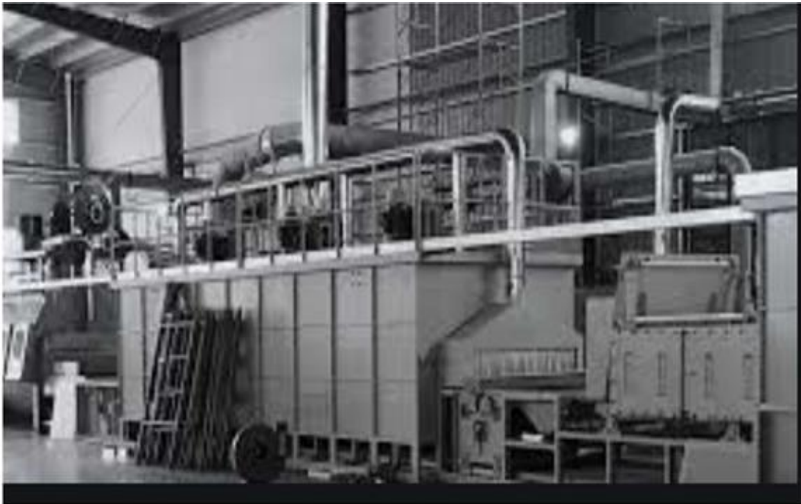
Industrial CAB Furnace
