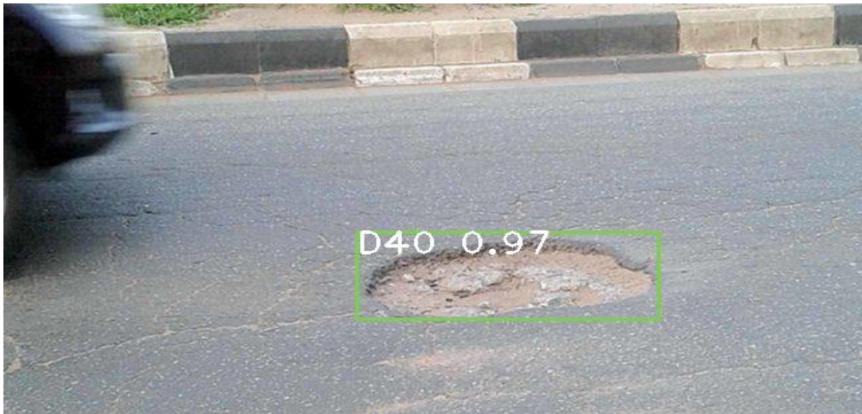
Figure 9: Detected Images of Potholes
