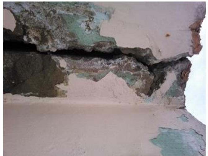
Figure 2-4 Expansion joint treated by improper materials (shotcrete and mortar)
