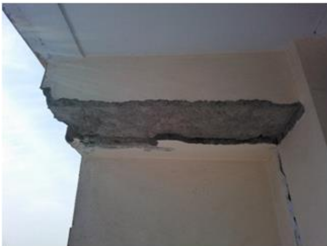
Figure 2-3 Beams nearby the joint, indicates pounding by unexpected ampules.
