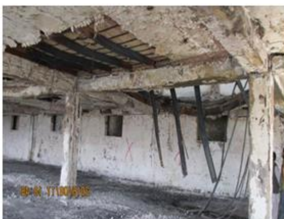
Figure 2-10 Demonstrations cracks on the column
