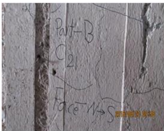
Figure 2-9 Shows cracks on the 21st column
